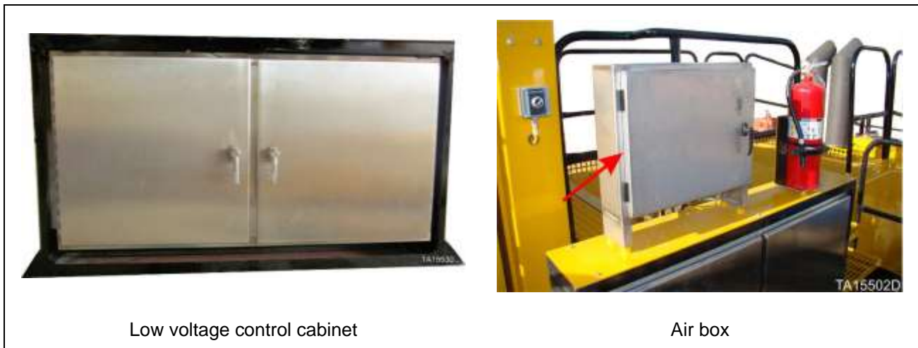
Figure 29. Low voltage control cabinet and air box typical locations
