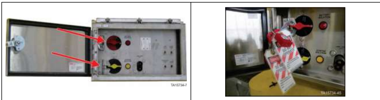
Figure 2. Battery Isolation Box – Battery isolation switch in OFF position with locks in place
